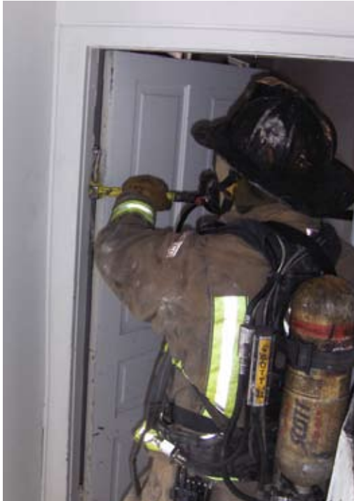
The adz is slipped in to the space between the door and the jamb near the hinge allowing it to easily be pried off.
